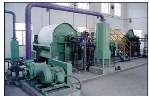
Drum Filter Vacuum System
